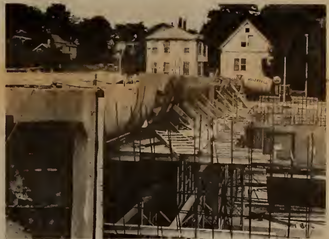
The site of the Boylston Street/Jamaica Plain station which has been prepared for the construction contract recently awarded.
